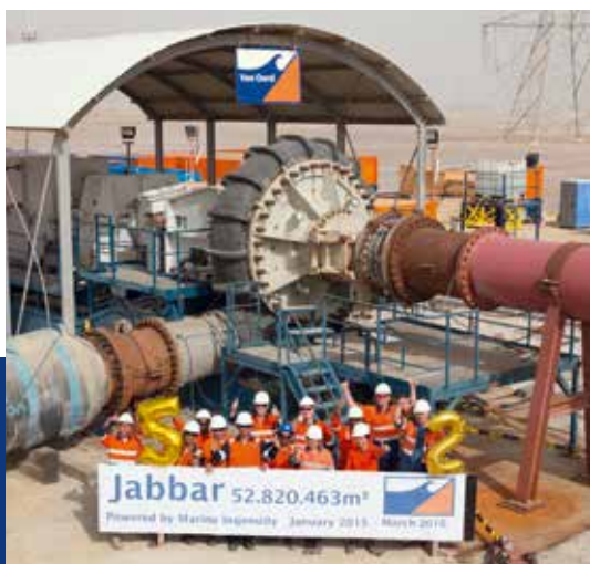
Innovative booster station Jabbar
