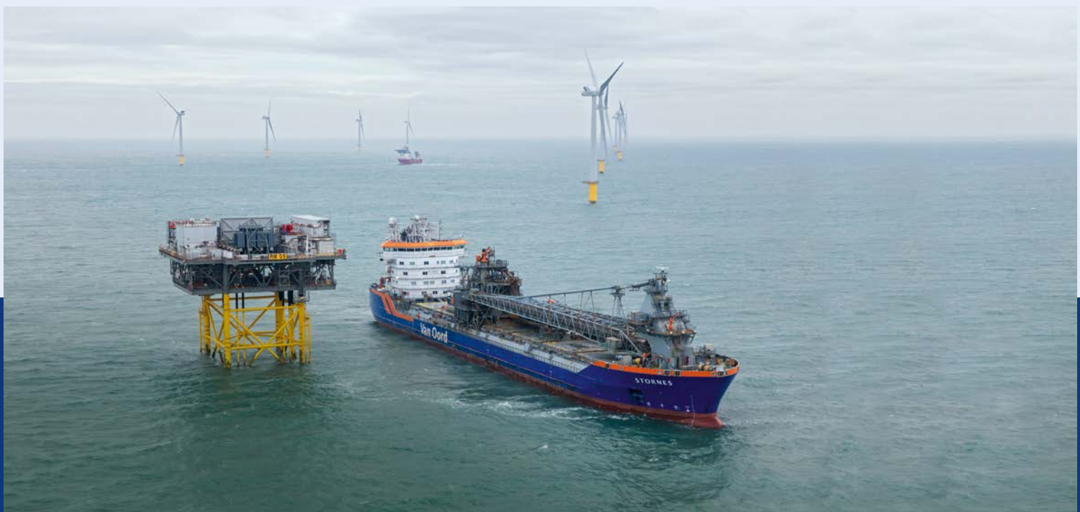
Flexible fallpipe vessel Stornes at work installing scour protection at the Rampion Offshore Wind Farm
