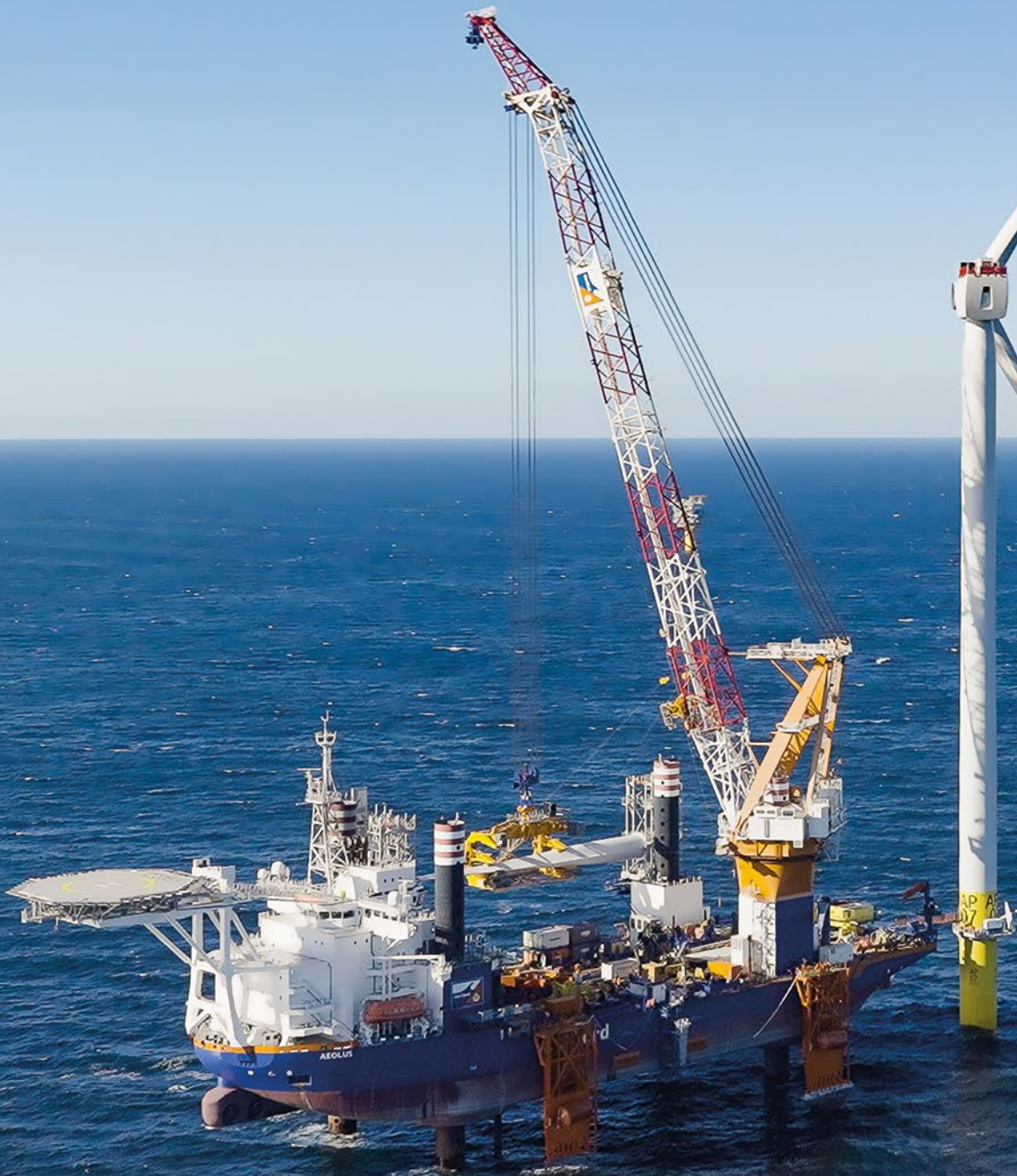
Van Oord's offshore installation vessel Aeolus installed 12 turbines at the South Fork offshore wind farm. The first offshore wind project in the US State of New York.
