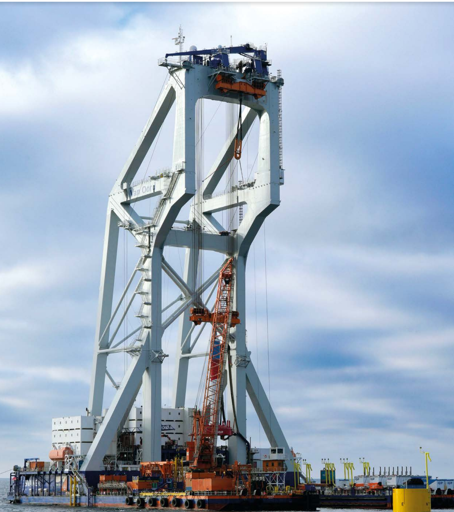
Heavy lift installation vessel Svanen installing the first monopile for the Baltic Power offshore wind farm. With a capacity of up to 1.2 GW, Baltic Power will eventually supply sustainable electricity to more than 1.5 million Polish households.
